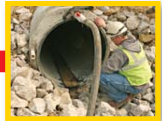
The grout is pumped into the entire length of the pipe, filling in all voids between the new and host pipe, and the areas between the pipe and roadway.
