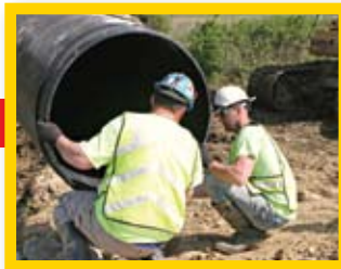
A gasket is installed on the next piece of pipe, assuring a watertight seal when connected, meeting ASTM D3212 requirements.
