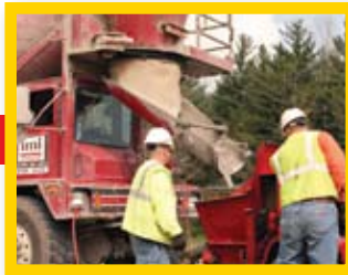
Workers prepare the low density cellular grout that will be pumped into the pipe.
