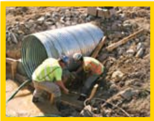
The same culvert, excavated and prepared for Snap-Tite® rehab. Since the pipe was so deteriorated, this project required the installation of a corrugated metal sleeve to accept the new pipe. A concrete footer was also poured.
