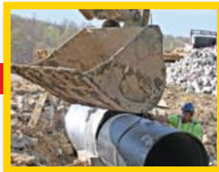
The first piece of Snap-Tite® HDPE is lowered into position and inserted into the host pipe.
