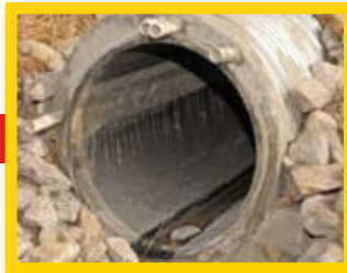
Different length PVC pipes that will deliver the grout flow are installed, and both ends of the pipe are sealed.
