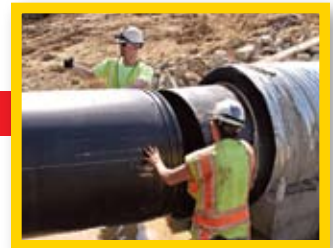
The second piece of pipe is lowered into position, and lined up with the first piece.
