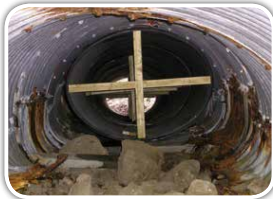
Snap-Tite® pipe coming through a deteriorating culvert during installation (struts will be removed once completed).
