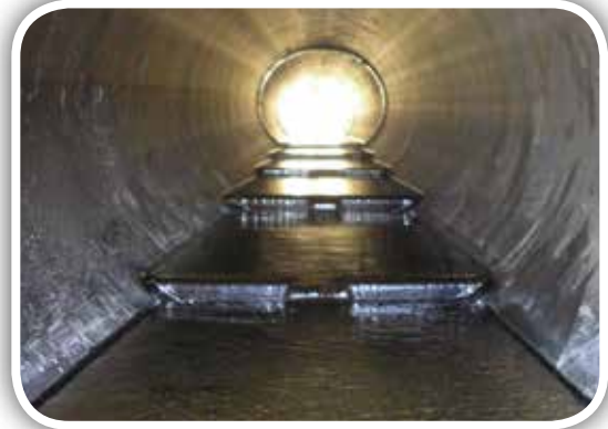
Ponding effect created by baffle/weir design during low-flow.
