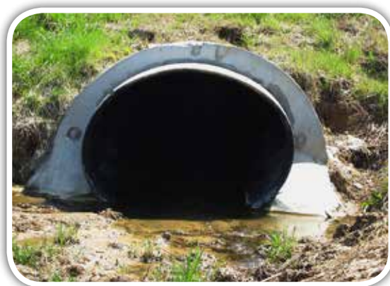
A culvert, rehabilitated with Snap-Tite® oval pipe.
