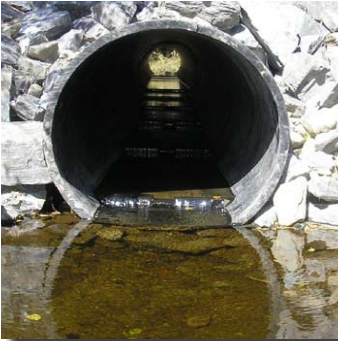
Pools adjacent to culvert can play important design elements in aquatic passage.
